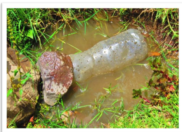
The new strainer in place, in a shallow capture basin
